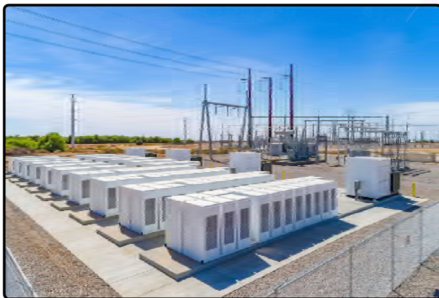
Battery Energy Storage System
