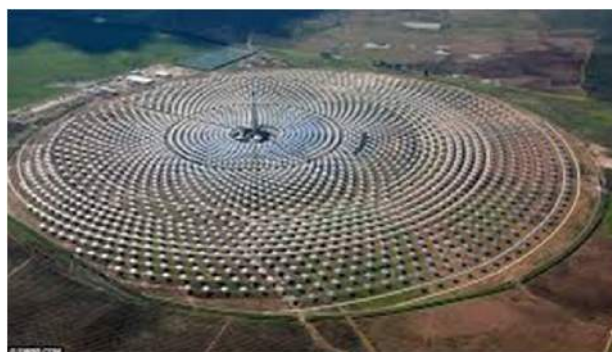
Figure 5 : Gemasolar Power Plant in Spain.
